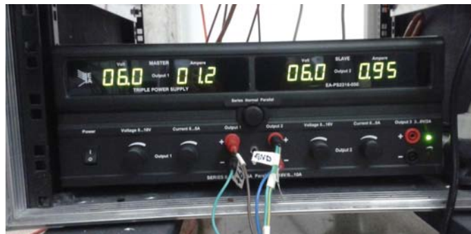
Power supply for converter
